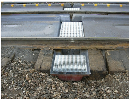
Crossdrain with Drain Cover
